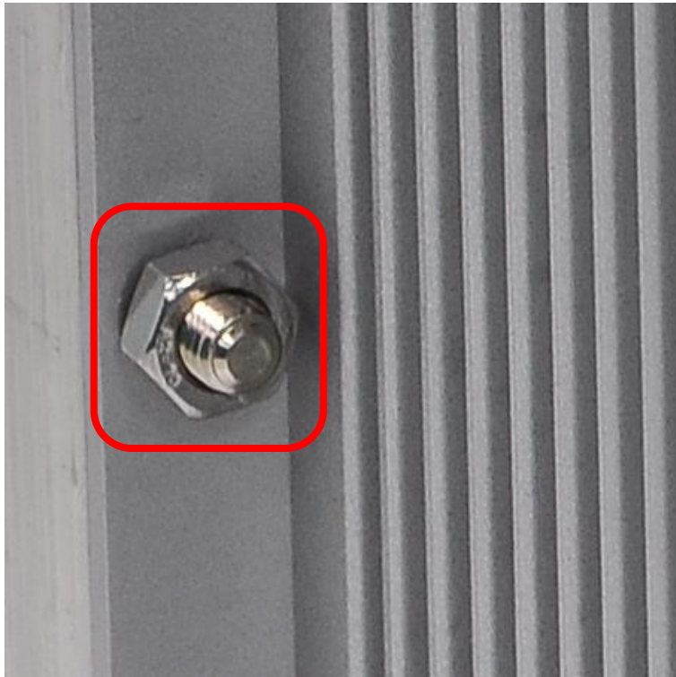
Ground screw of the switch
