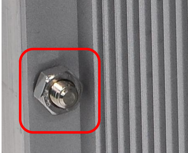
Ground screw of the switch
