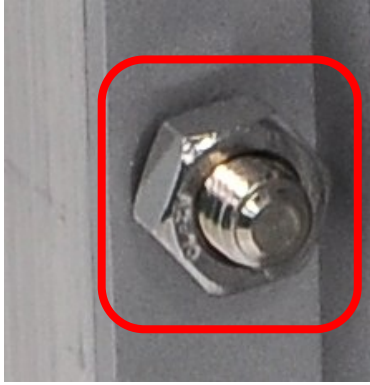
Ground screw of the switch
