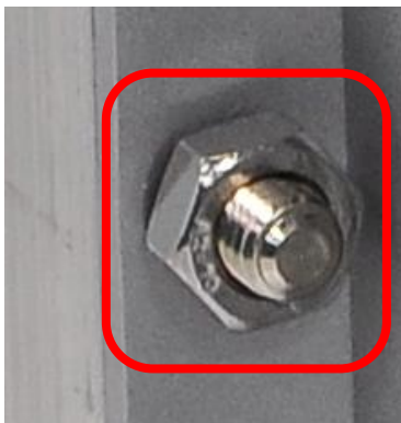
Ground screw of the switch
