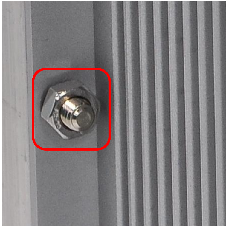
Ground screw of the switch
