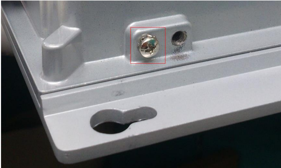
Ground screw of Ethernet switch
